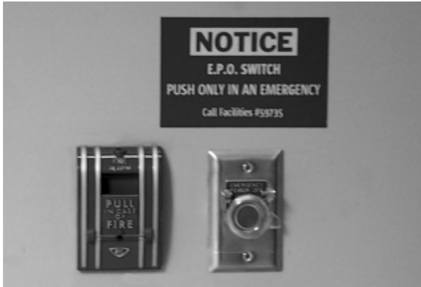
FIGURE 7-4 Emergency Power Disconnect and Manual Fire Alarm Pull Station
