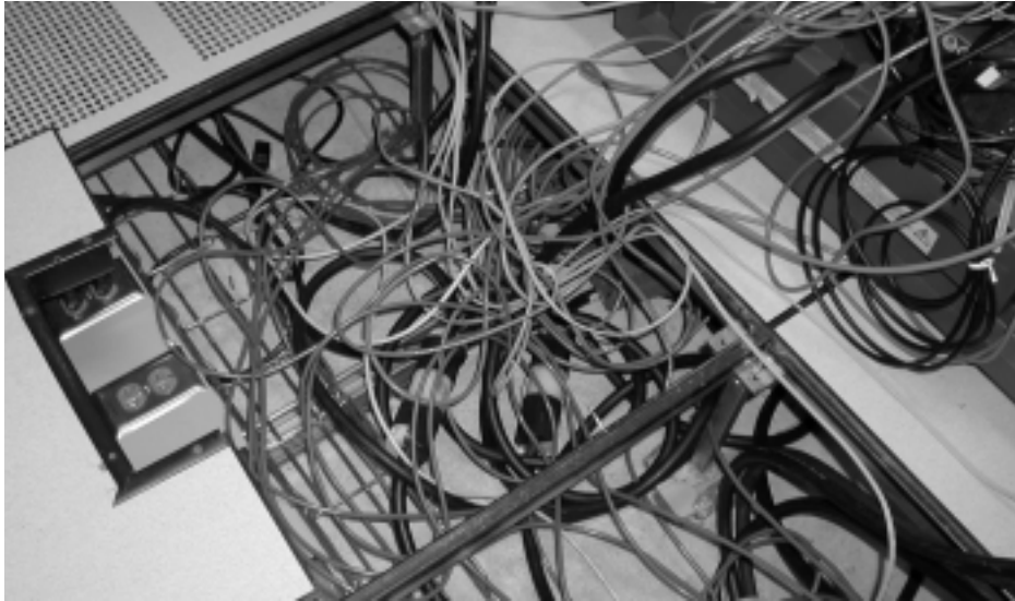
FIGURE 7-5 Disorganized Cabling Under Floor Tiles
