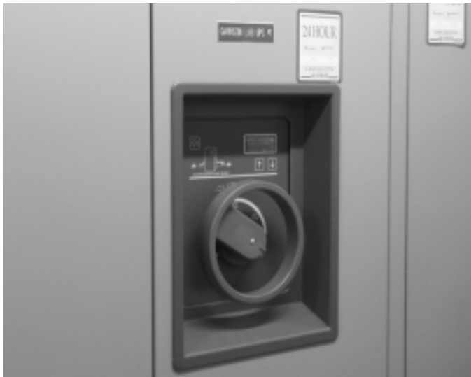
FIGURE 7-1 Control Panel and Digital Display of a UPS System
